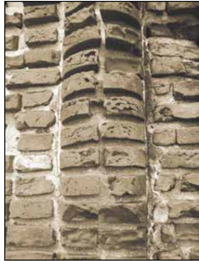
Close-up of the half-columns of brick, showing the use of pie-shaped bricks to achieve the curved shape.
