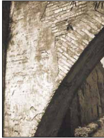
Lower part of the solid brick arch that supported the choir loft.
