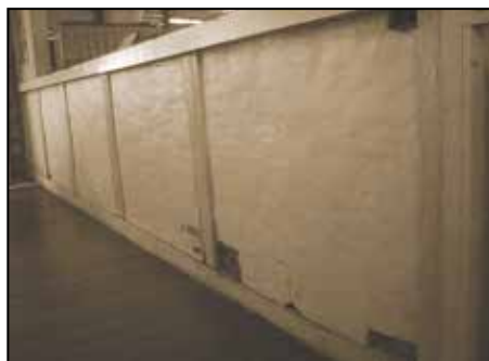
Fig. 15. Portion of half-wall of tabique pampango in the convento of Dapitan, Zamboanga del Norte.
