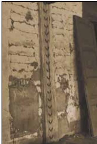
Fig. 28. Closer view of the upright frame post with diagonal slots for the horizontal boards.
