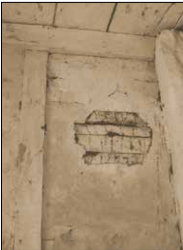
Fig. 18. Detail of tabique pampango wall in ground floor of convento, Dauis, Bohol.
