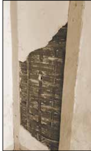
Fig. 6. Detail of plaster peeling over wattle.
