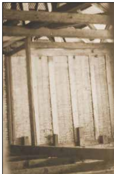
Figs. 30, 31, 32. Two types of tabique pampango in convento of Loboc, Bohol (before the 2013 earthquake).
