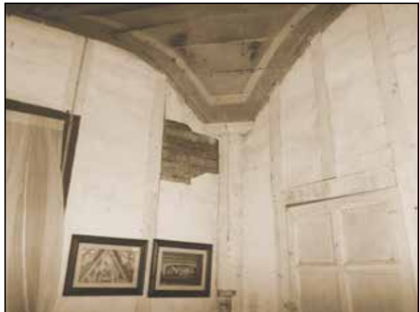
Fig. 19. Detail of tabique pampango wall in main hall in upper level of convento, Dauis, Bohol.
