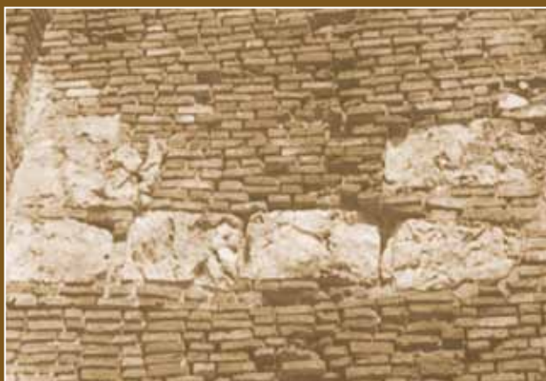
Detail of the wall at the back of the church in Batac. Coral-stone blocks, most probably from Paoay, were inserted to replace bricks that had broken loose.
