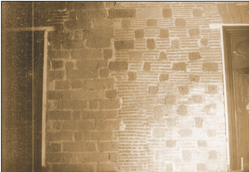
Section of the inner wall of the convento , showing the earlier construction (brick and stone) and the later one just of stone
