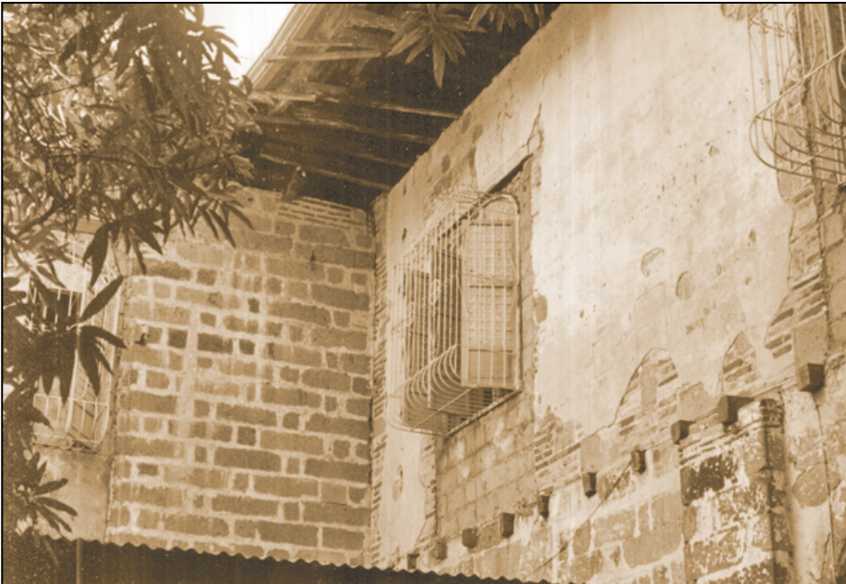
Portion of the exterior wall of the convento . The palitada (protective lime plaster) on the second floor has been retained, but where it has fallen off, the checkerboard pattern of brick and stone can be seen. The opposite wall of cut stone pertains to the 19th century extension of the convento
