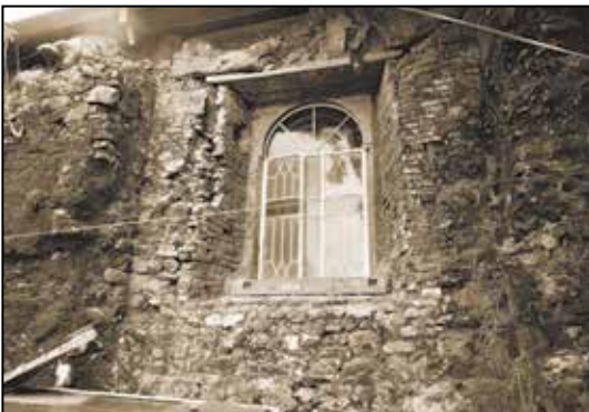
Window of the right side of the church, showing brickwork over earlier rubblework wall.
