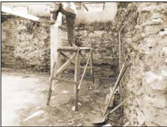
A room in the ground level of the convento, showing different states and construction techniques of the brick wall.
