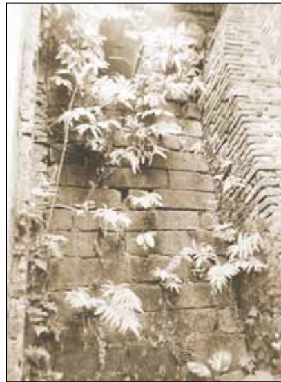
A cut-stone wall connects the tower and the back of the façade.
