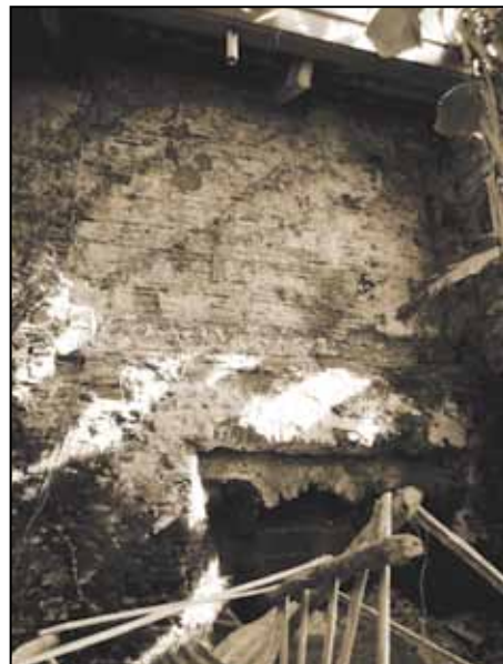
North wall of the church towards the façade. It still retains the original paletada lime plastering. In the lower section is the doorway, now sealed, which connected the church with the convento.
