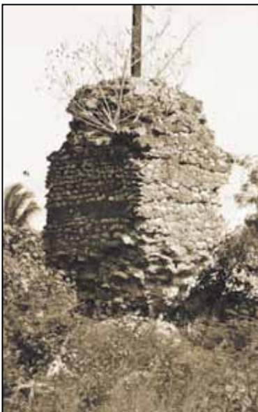
One of the masonry pillars in the apse now supports a cross, but its lower portion is in danger of collapse.
