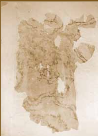
A portion of paint in the transept has peeled off, revealing an earlier "marbling" effect.
